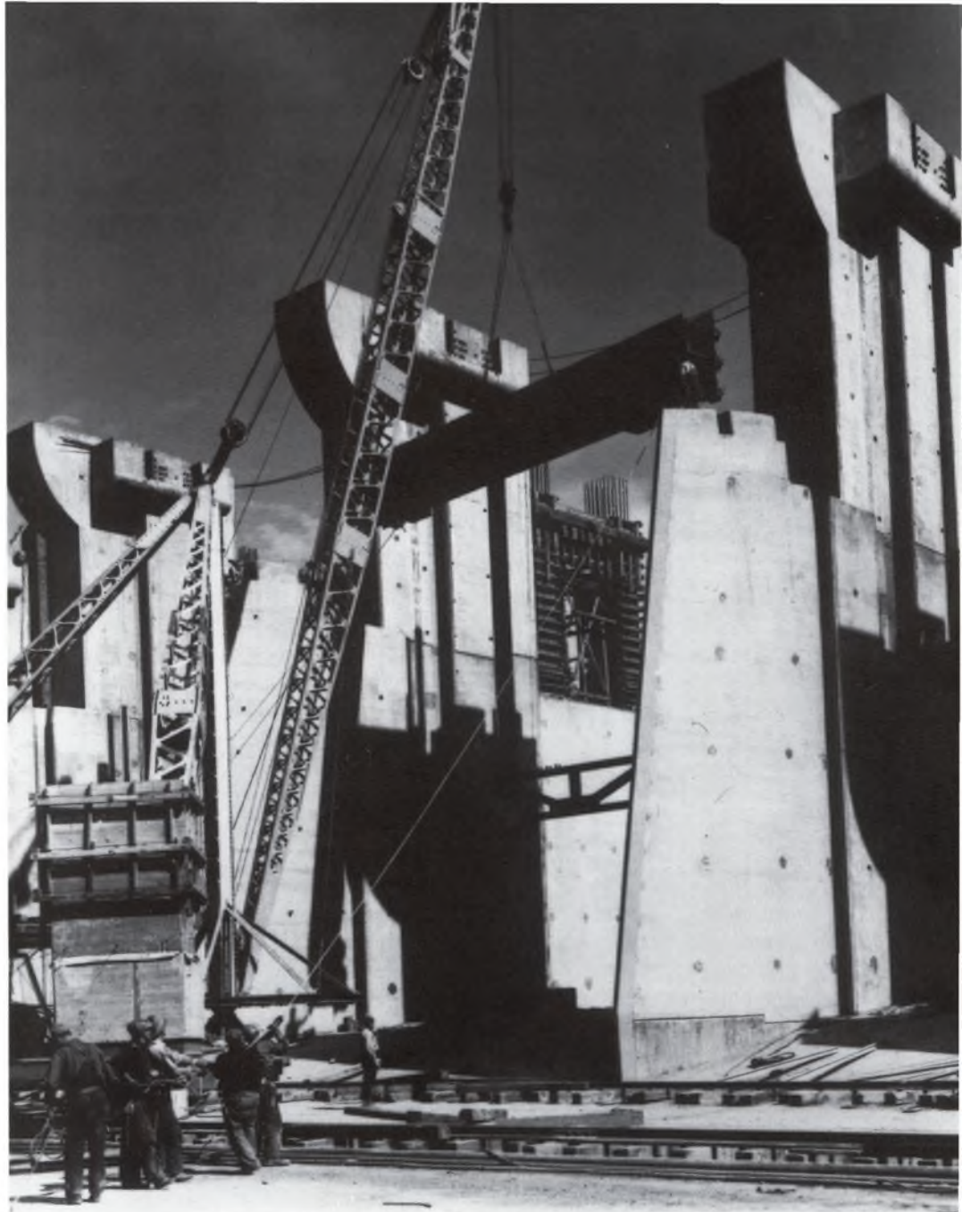
Fort Peck Dam – spillway gate construction. June 10, 1937. Photograph used with the permission of Montana Historical Society, Helena. Photo: U.S. Army Corps of Engineers.
